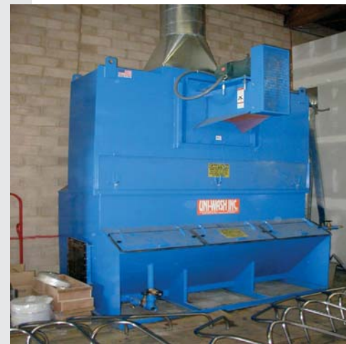
UNI-WASH Model UCBD-75 7,500 CFM Wet Type Dust Collector installed on a grinding operation
