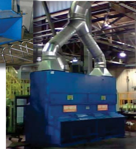
UNI-WASH Model UCBD-100 10,000 CFM Wet Type Dust Collector installed on a forging operation
